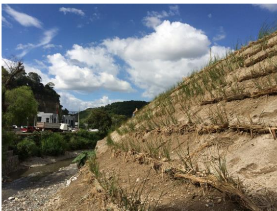
Figure No. 6. Soiltraps working at fill slope. Kindly by Vetiver te, Guatemala.
