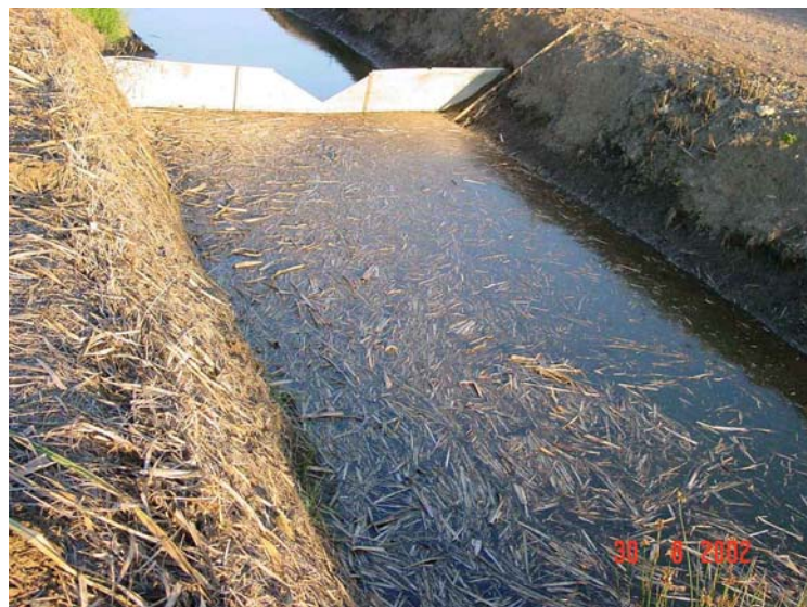
Photo 8. Impact of cane trash on control section of drain after harvesting.
