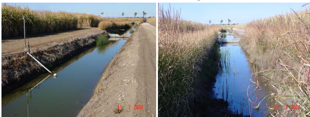
Photo 4: Exposed and highly erodible banks of the control section (left) as contrast to the well stabilised section of the trial (right).
